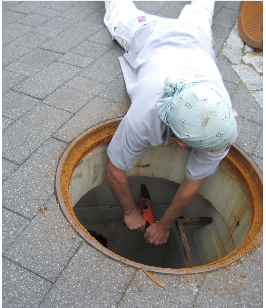
Figure 25. Installation of the Pressure Transducers at the Overflow of the Cistern (Credit: Emily McCoy)
