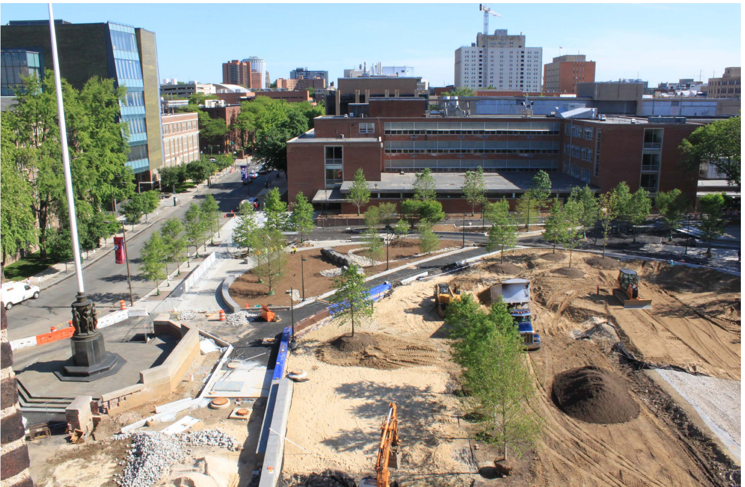
Figure 5. Soil during Construction: Engineered soil being placed at Shoemaker Green, University of Pennsylvania, Philadelphia (Credit: Andropogon Associates)
