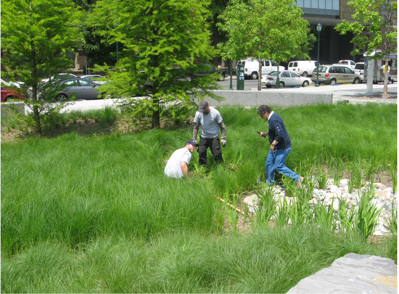
Figure 26. Installation of the Automatic Sampler Intake at the Bottom of the Rain Garden (Credit: Emily McCoy)
