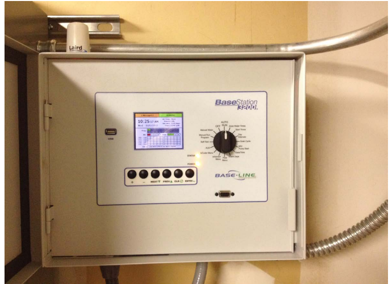
Figure 12. Irrigation Controller (Credit: Emily McCoy)
