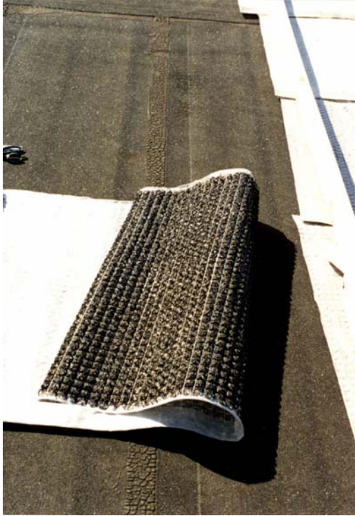
Figure 3. Drainage cloth: a component of a “loose-laid” or “built-up” system. Location: San Bruno, CA. Source: McDonough + Partners
