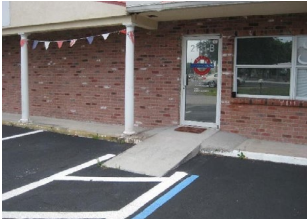
Figure 37. Non-conforming ADA ramp; no handrails (vertical rise exceeds 6"); no door landing to accommodate wheelchair and door swing; ramp protrudes into aisle. Applicable ADA 2010 Code Standards: 405 (whole section), 502.4, 404 (whole section), 505 (whole section), 603.2
