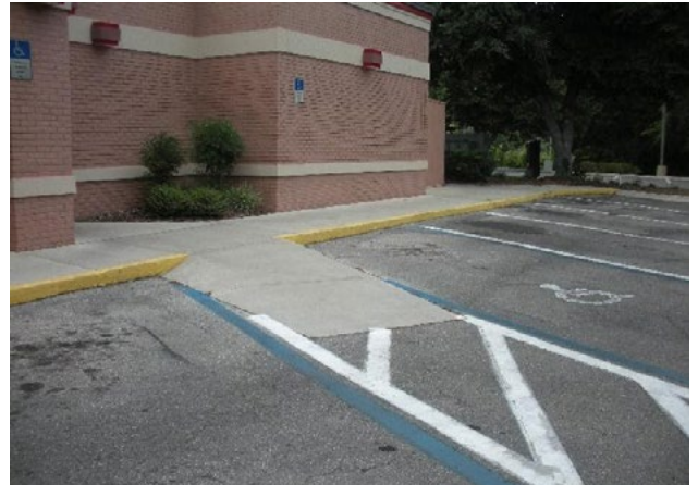
Figure 32. Curb ramp located in required ADA access aisle; hazardous side slopes. Applicable ADA 2010 Code Standards: 406 (whole section), 502 (whole section)
