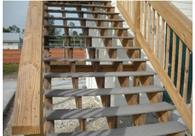
Figure 50. Open risers; lack of accessible handrails. Applicable ADA 2010 Code Standards: 504.3, 505 (whole section)
