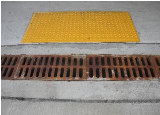
Figure 51. Catch basin grate in accessible route; gaps too wide on grate. Applicable ADA 2010 Code Standards: 302.3
