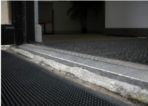
Figure 49. Nonconforming threshold height creating significant barrier and trip hazard. Applicable ADA 2010 Code Standards: 404.2.5, 404.3.3
