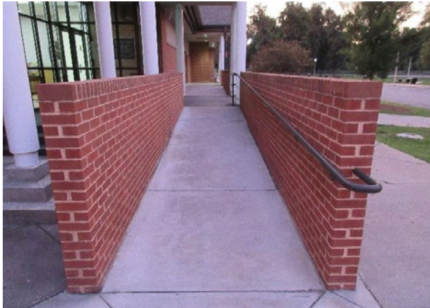
Figure 25. Ramp handrails not provided on both sides of ramp. Applicable ADA 2010 Code Standards: 505 (whole section)
