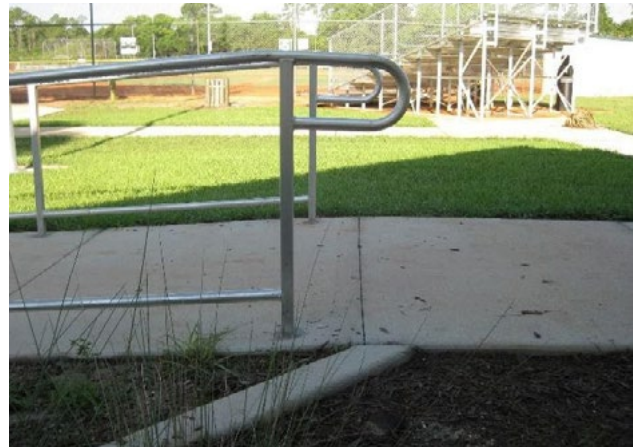
Figure 28. Ramp handrails don't extend far enough past the top of slope, no edge protection on ramp. Applicable ADA 2010 Code Standards: 405.9, 505.10
