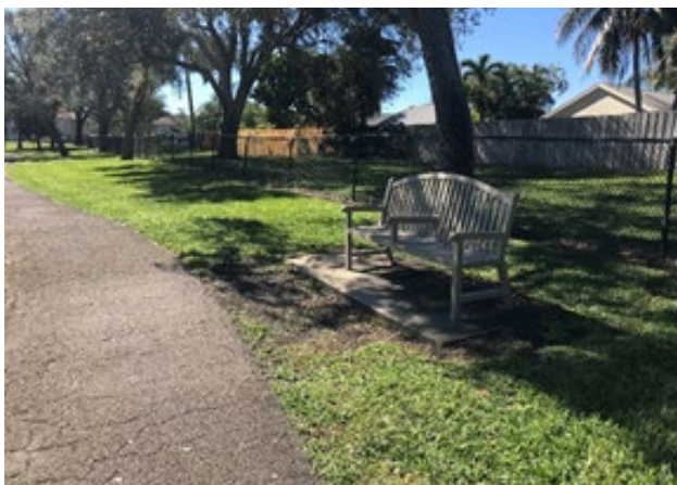
Figure 41. No clear ground space for wheelchair on accessible route and adjacent to bench (ABA). Applicable ABA Standards: 1011
