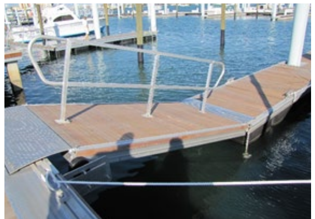
Figure 42. Many exceptions exist for gangways, but must have handrails both sides and edge protection. Applicable ADA 2010 Code Standards: 1003.2
