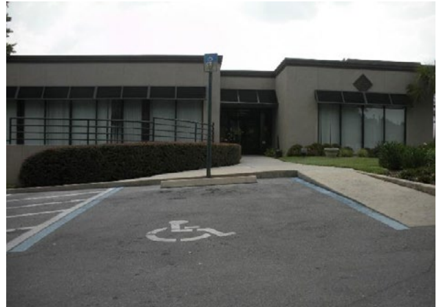
Figure 38. Access aisle not on same side as curb ramp (not on accessible route); parking clear zone; space and aisle exceed allowable slope. Applicable ADA 2010 Code Standards: 402.1-403.4, 502 (whole section)
