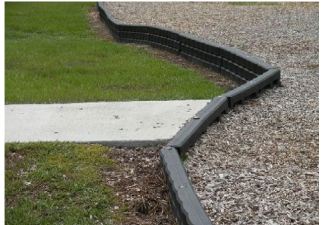
Figure 22. No accessible route into playground. Applicable ADA 2010 Code Standards: 1008.2
