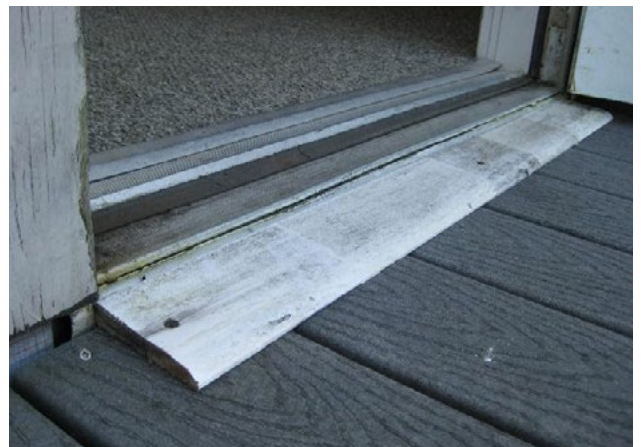
Figure 30. Nonconforming threshold height and configuration (deck elevation set too low). Applicable ADA 2010 Code Standards: 404.2.5
