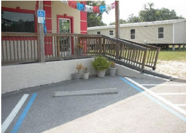
Figure 43. Excessive ramp slope; no accessible handrails. Applicable ADA 2010 Code Standards: 405 (whole section), 505 (whole section)
