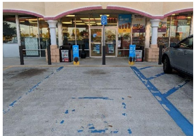
Figure 48. Nonconforming sign; inadequate area, striping; accessible route blocked. Applicable ADA 2010 Code Standards: 402 (whole section), 502 (whole section)
