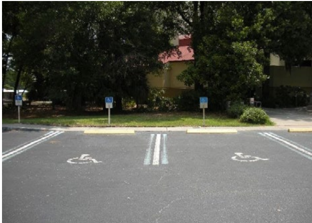
Figure 19. ADA signage incorrect height; lack of aisles. Applicable ADA 2010 Code Standards: 208.3, 502 (whole section)
