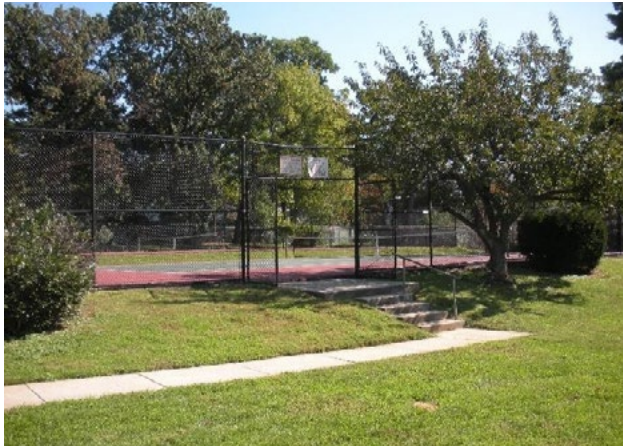
Figure 31. Lack of accessible route to sport courts although ramp would be readily achievable. Applicable ADA 2010 Code Standards: 402 (whole section), 206.2.12
