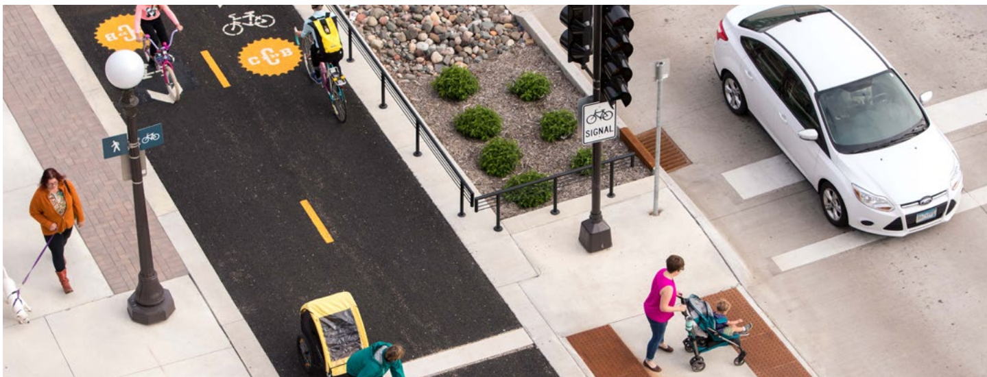
Jackson Street Reconstruction, Saint Paul, Minnesota, Toole Design / Toole Design. (Image Credit: Bruce Buckley Photography for Toole Design)
