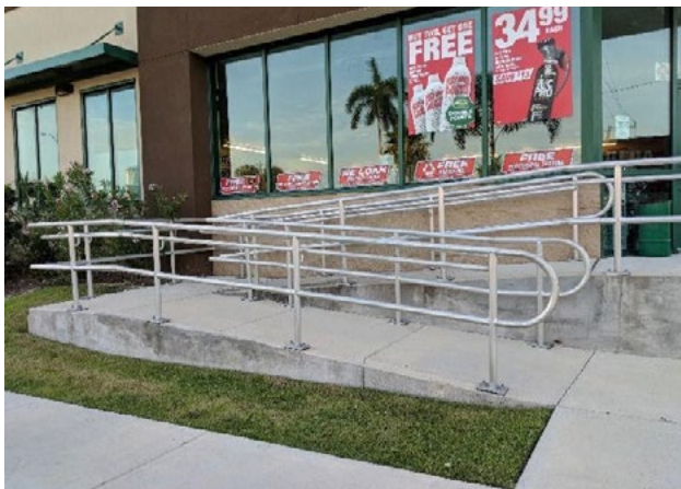
Figure 23. No handrail extension beyond ramp; no ramp edge protection. Applicable ADA 2010 Code Standards: 405.9, 505.10
