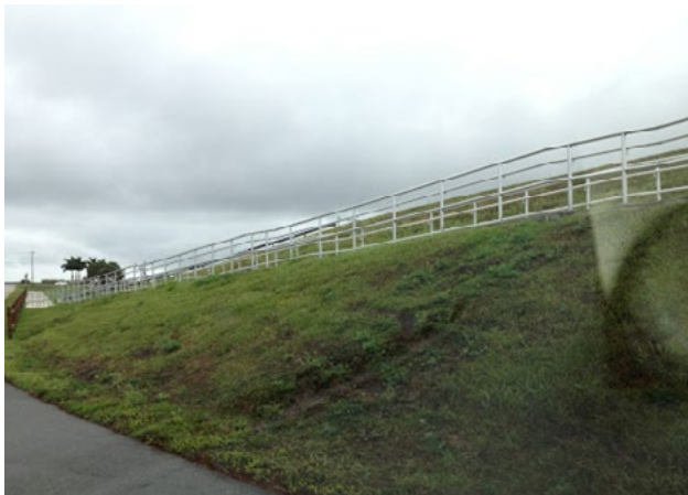
Figure 15. Even a long ramp can meet requirements for run lengths and landings
