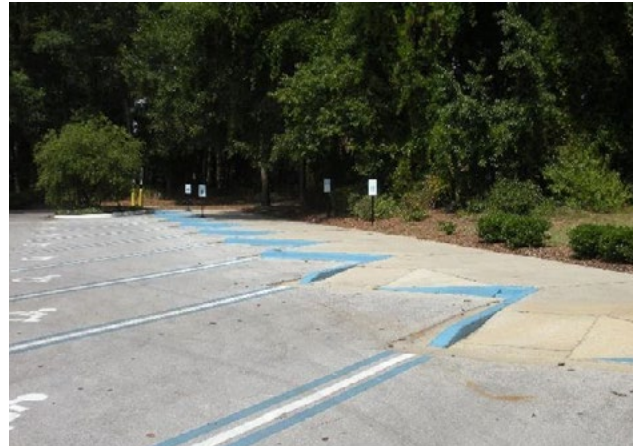
Figure 44. Lack of access aisles and signage. Applicable ADA 2010 Code Standards: 402 (whole section) 502 (whole section)
