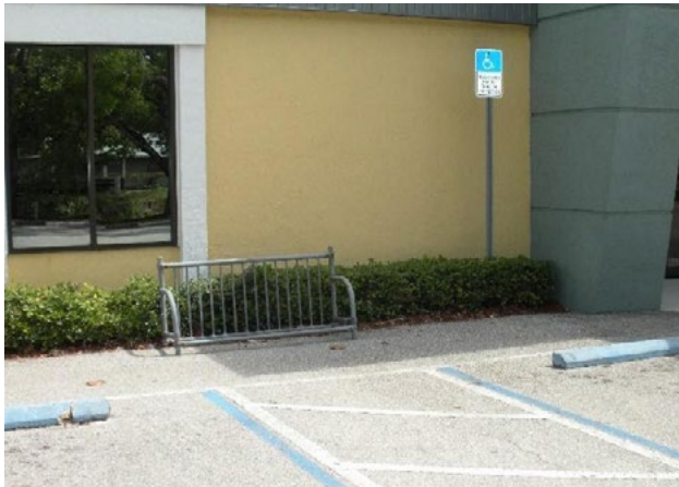
Figure 27. Bike rack at accessible aisle creates obstruction in accessible route. Applicable ADA 2010 Code Standards: 403.5
