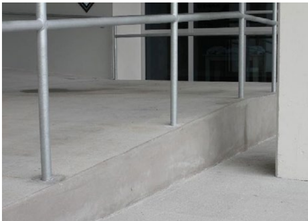
Figure 39. No ramp edge protection. Applicable ADA 2010 Code Standards: 405.9
