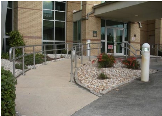
Figure 33. Handrails do not extend far enough; slopes and landings out of compliance; curved ramps not recommended due to complexity of compound slopes. Applicable ADA 2010 Code Standards: 405 (whole section), 505 (whole section)
