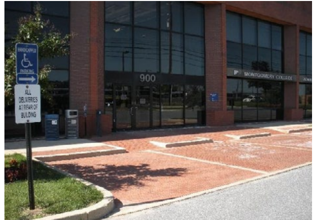
Figure 20. Inappropriate ADA parking signage; no access designated access aisles. Applicable ADA 2010 Code Standards: 502 (whole section)
