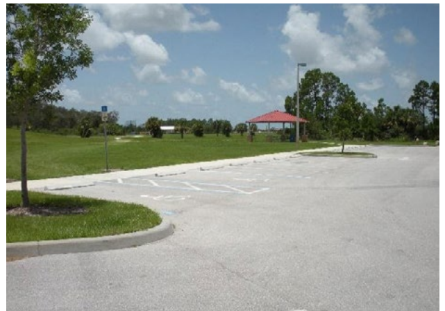
Figure 34. ADA parking not located on shortest cross route to destination (pavilion). Applicable ADA 2010 Code Standards: 208.3
