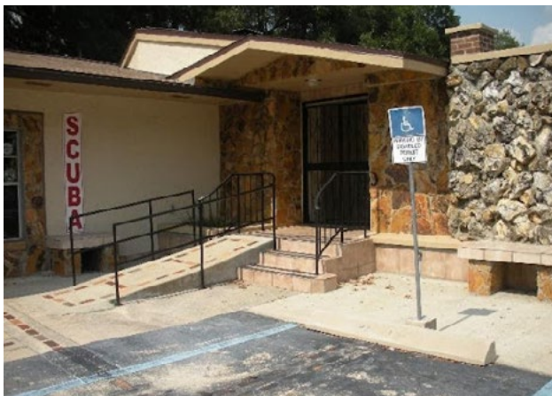
Figure 53. No accessible aisle striping; excessive ramp slope; no handrail extensions on steps or ramp, sign within overhang. Applicable ADA 2010 Code Standards: 405 (whole section), 502 (whole section), 505 (whole section)
