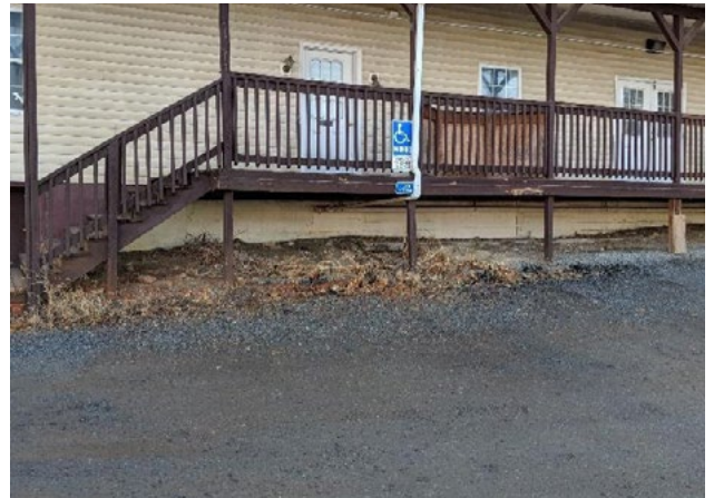
Figure 52. No ADA parking space or aisle striping; no accessible route to entrance. Applicable ADA 2010 Code Standards: 402 (whole section), 502 (whole section)
