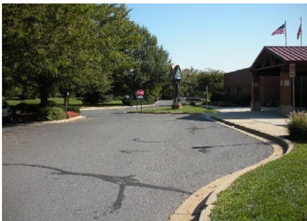
Figure 35. No marking of loading/unloading zone or access aisle. Applicable ADA 2010 Code Standards: 503 (whole section)
