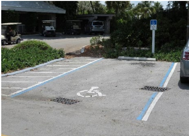
Figure 21. ADA parking access aisle does not connect to an accessible route. Applicable ADA 2010 Code Standards: 502.3
