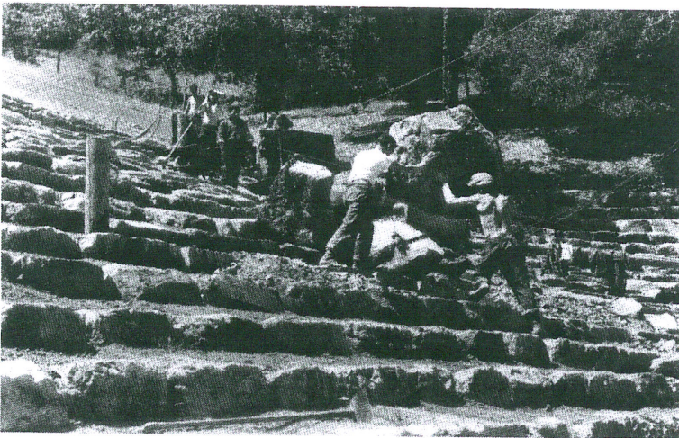
FIGURE 43. 1937. Per Knight's instructions, workers selected stones with two surfaces at right angles to provide a flat top and vertical riser without compromising the weathered look of the stones by cutting them (NA).
