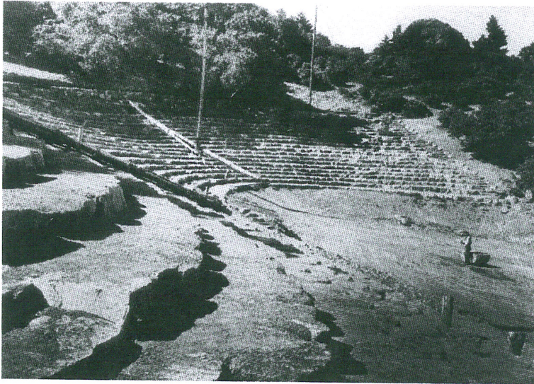
FIGURE 42. c. 1937–1938. Upon completion of the lower 20 rows, the 80-foot high booms were relocated to the top of the theatre and a track rail was installed along the middle aisle to distribute stone across the site more quickly (UCCEDA).
