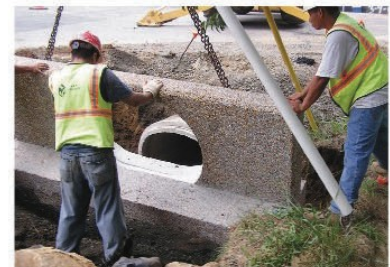
Cost-effective solutions for reducing the visual contrast of concrete included the use of exposed aggregate and a slight tint to take away the bright white look of all exposed concrete surfaces
