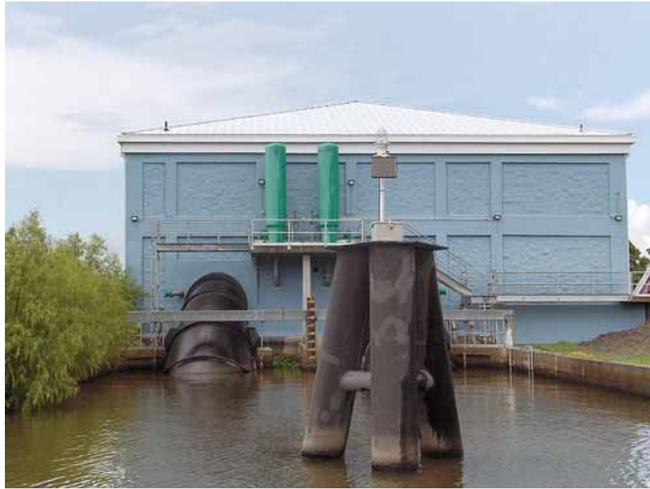
Typical pump station in New Orleans. Canals are used to direct stormwater into these energy-intensive pump stations, which discharge stormwater over protective levees into adjacent waterways during storm events.
