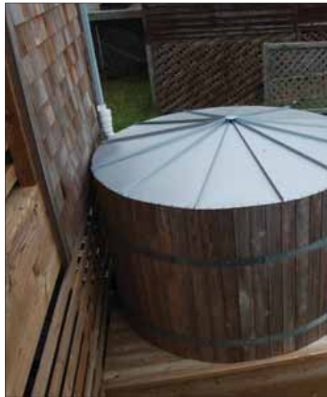
Rainwater collection systems allow for reuse of captured water and reduce the amount of runoff entering the municipal drainage system. (photograph by Flickr.com user BOBXNC under a Creative Commons license for usage)
