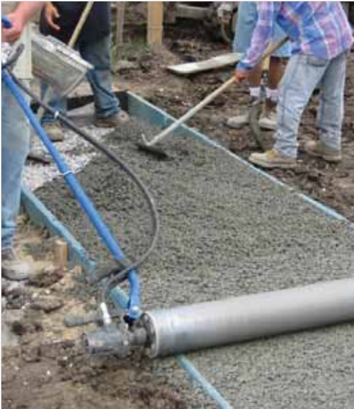
Installation of a pervious concrete sidewalk within the Make It Right project area in the Lower Ninth Ward. (photograph by Make It Right)
